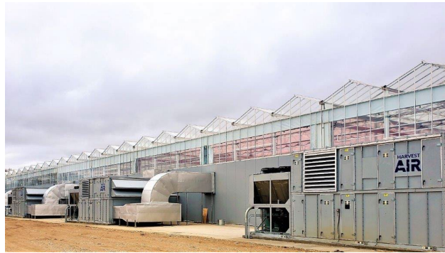
Sealed Greenhouse with Advanced HVACD Equipment
