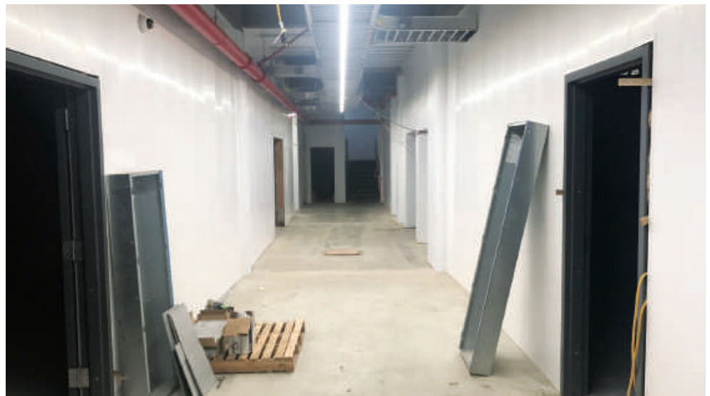
In this retrofitted facility, additions of easily cleanable PVC wall coverings and steel doors were used to increase cleanliness in the facility, while electrical infrastructure expansion allowed for proper mechanical systems to be installed.
